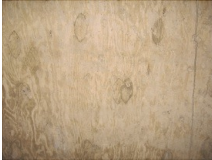
Fig. 9 Plywood knot marks left on today's poured concrete
