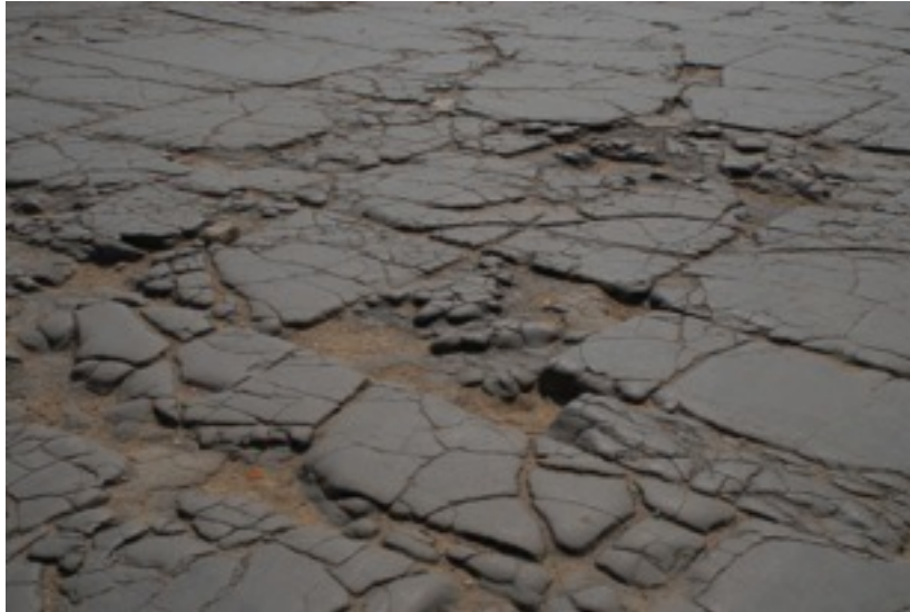
Fig. 6 Basalt platform near the NE corner of the Great Pyramid with cracks due to bad casting
